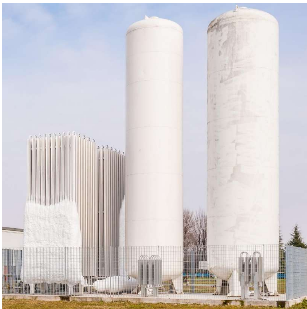
Picture no. 19: Cryogenic tanks.
